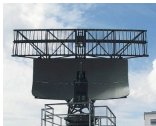
Figure 2: A monopulse secondary surveillance radar antenna (looks like a lattice fence) mounted on top of an antenna of a primary radar (parabolic reflector)
